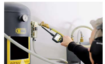
Leak detection with focus tube
