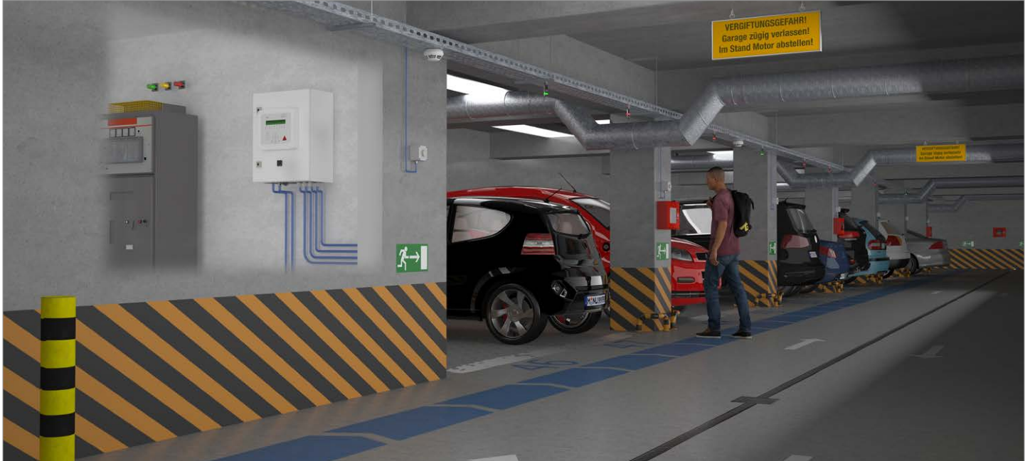
Example of a SCENTY® Gas Warning System in an underground car park
